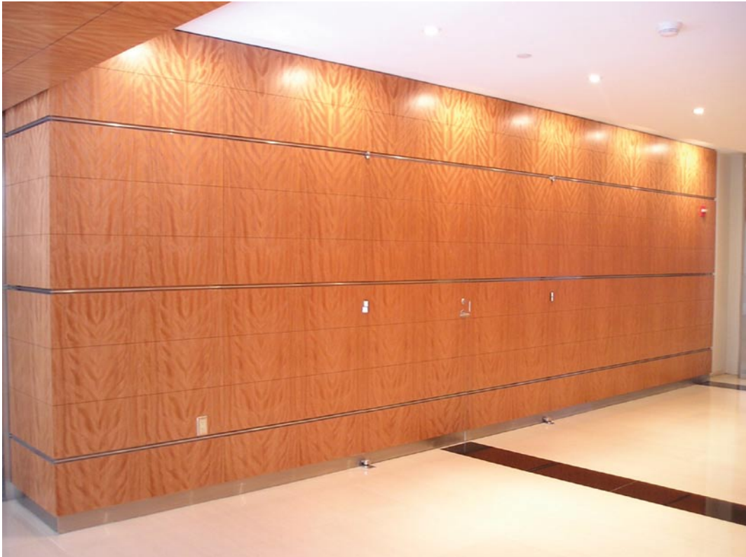
Example of "AA" grade blueprint matched installation.
